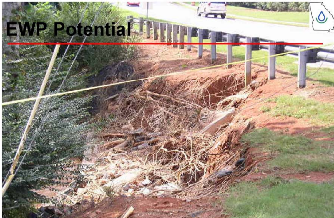
Damage at Taylor Road Downstream of Yellow River 16 in Gwinnett County. Without the watershed structure, this road would have been completely washed out. Some 3,750 bridges exist below NRCS structures in Georgia. Many were protected by NRCS dams.
