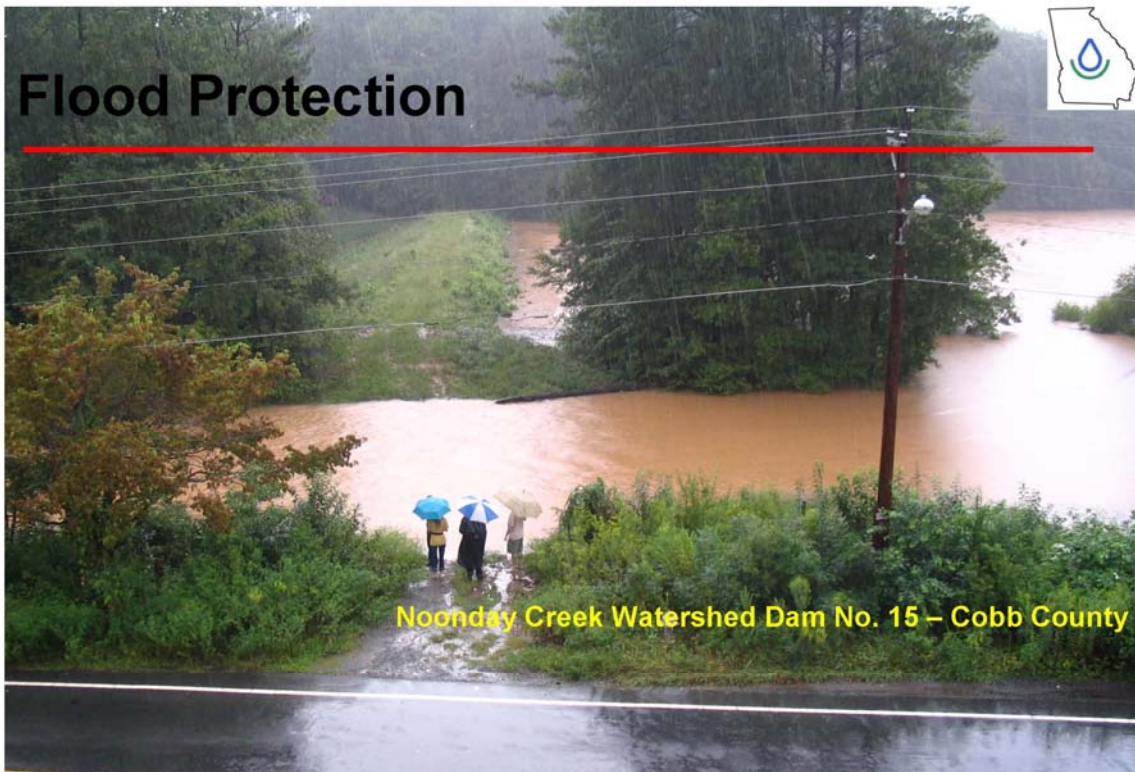
Working as Designed--Flow through the Auxiliary Spillway. This site is at Kennesaw State University with over 100 people working in offices within 300 yards below the dam.
