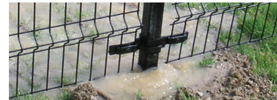
Sprinkler head is buried and can not pop up to properly water the lawn
